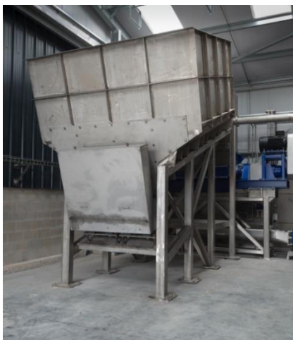
Raw material and Crusher
