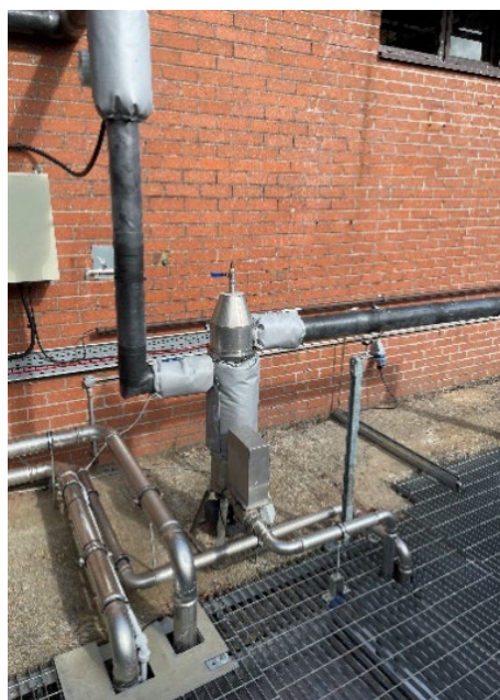
Pre filter stage taking water from the waste water pit
