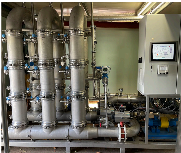
NanoPulse Waste Water Recycling system
