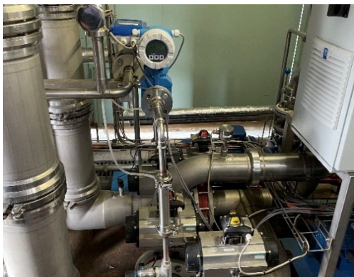
The 1" membrane test loop installed at JSG
