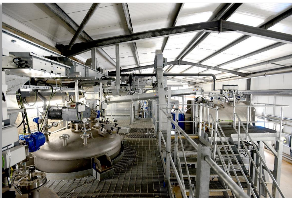
Fig 1. Reactors, materials handling, mixer
