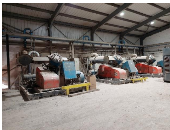
Figure 5: Interior of compressor house at Caudon
