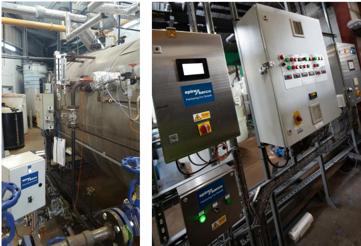
Figure 5: Picture showing the ITCS and instrumentation panels installed on the steam boiler at Bakkavor Wigan
