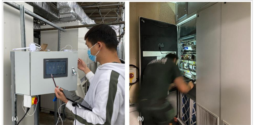
Figure 4 Demonstrator test runs: (a) UHULL researcher adjusting the demonstrator settings, (b) an engineer adjusting the existing air conditioners
