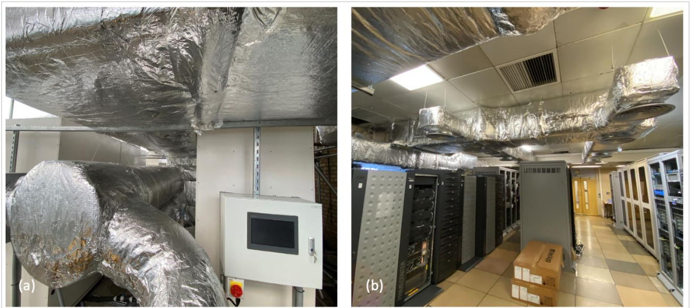
Figure 2 (a) External ducts and coolers, (b) internal ducts and servers
